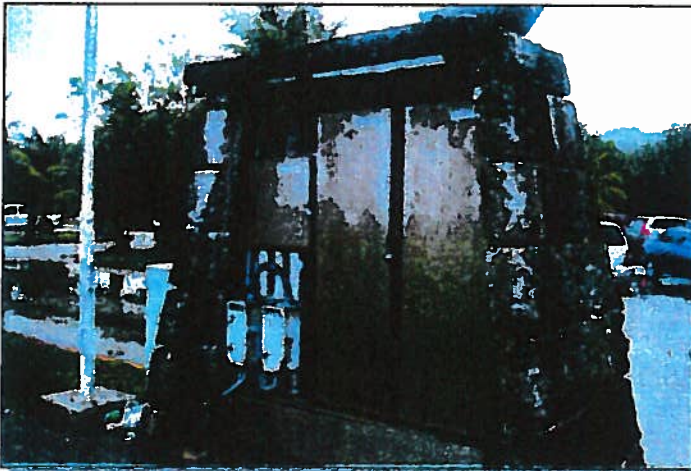
Electrical Panel Box
